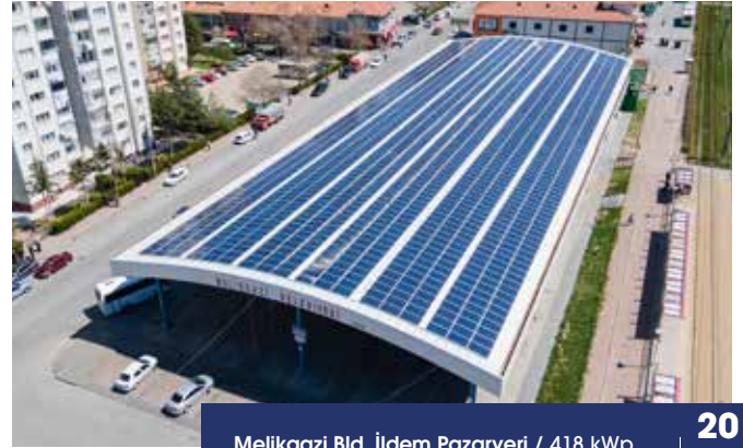
Melikgazi Bld. İldem Pazaryeri / 418 kWp
